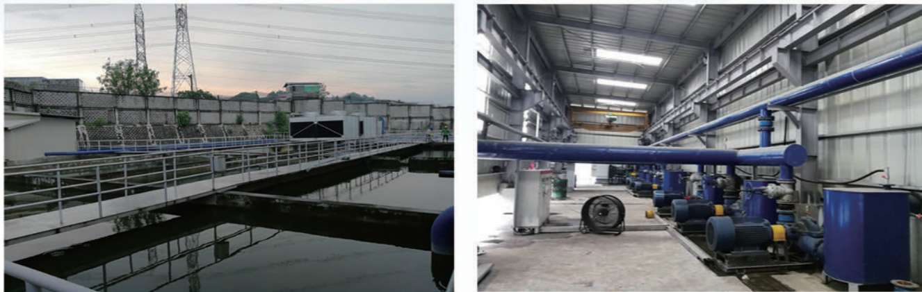
水池处理-水泵房 Water Pool Treatment - Water Distribution Pump Room
