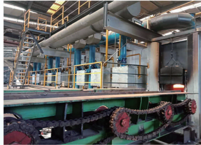
加热炉出口 Reheating Furnace Exit
